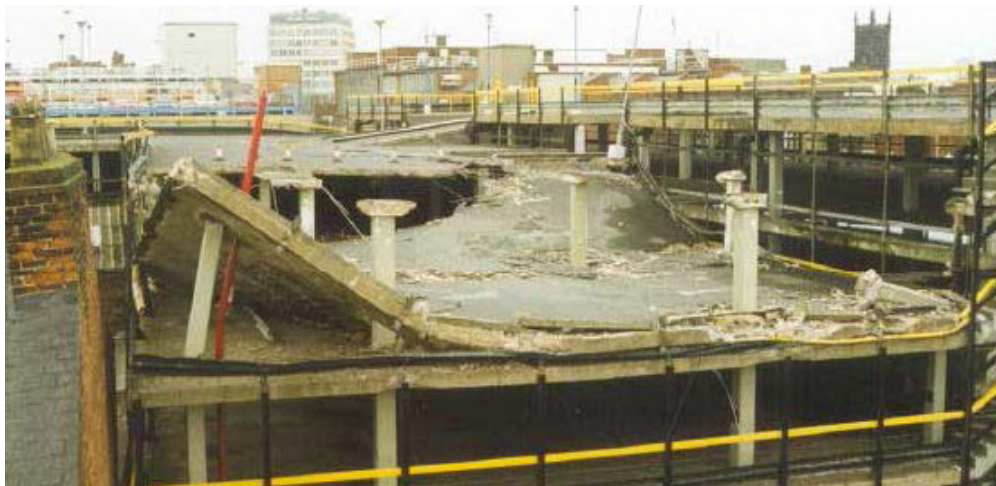
Pipers Row car park, Wolverhampton in 1997. Partial collapse attributed to carbonation and a lack of waterproofing to cracks https://www.hse.gov.uk/research/misc/index.htm
